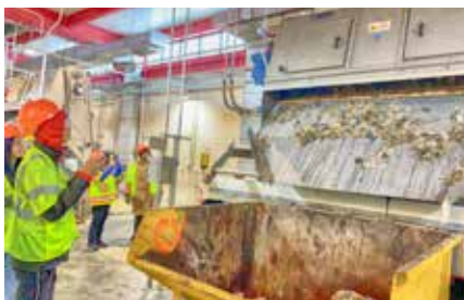
Wipes on bar racks at Southerly Wastewater Treatment Plant
